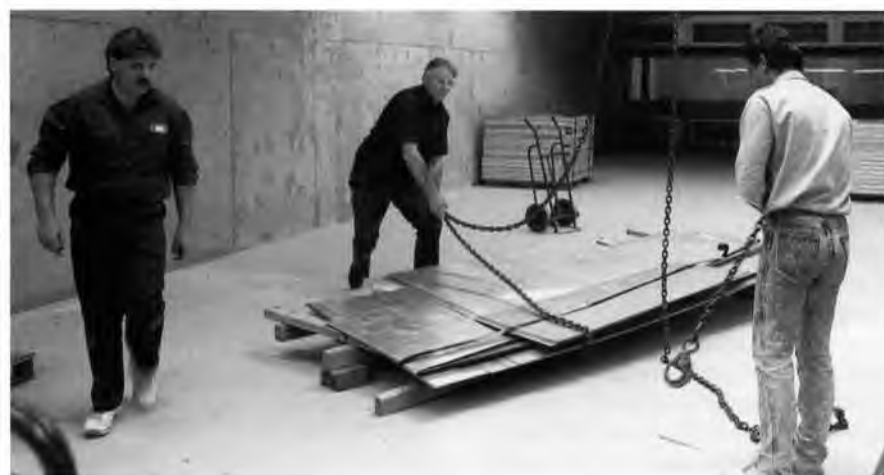
Sergeant Eric Riley, centre, lends a hand as components for the range are lowered through the roof of the Melbourne HQ building.
