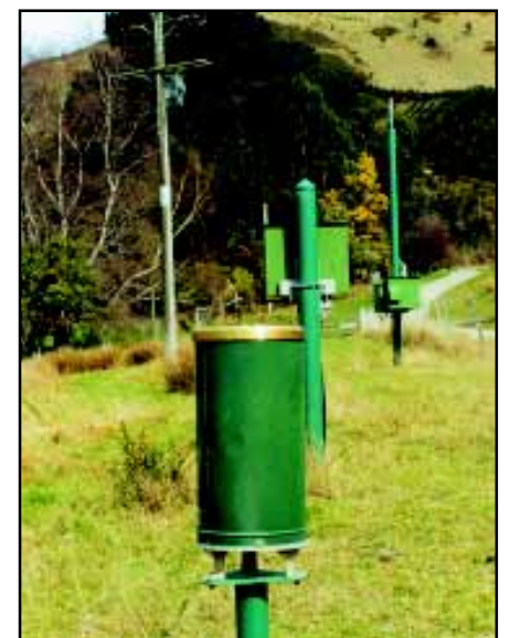
Figure 3: Telemetered rain gauge site at Blandswood
