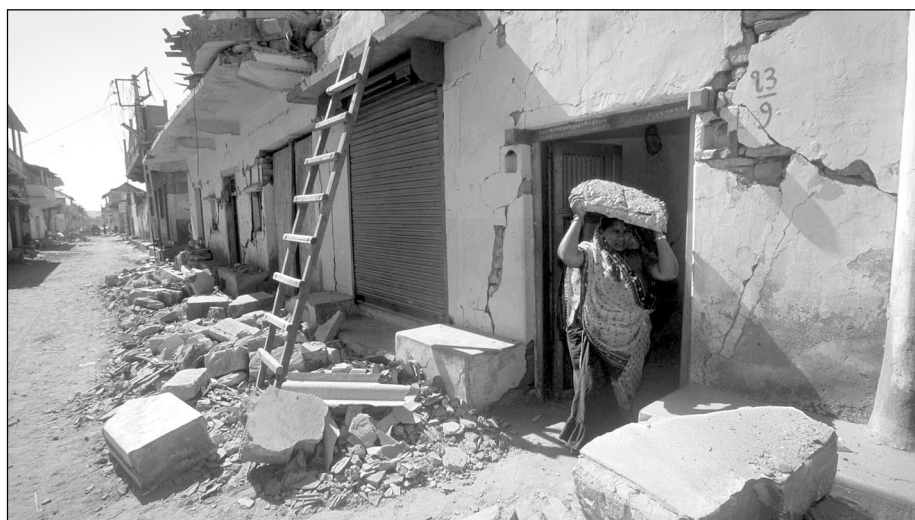
top: In El Salvador, many homes were lost beneath a wall of debris from a collapsing slope above. above: In Gujarat, the earthquake didn't kill, but the buildings did. (images courtesy International Federation of Red Cross and Red Crescent Societies)
