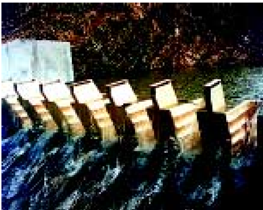
Top: Fuseplug emergency spillway. Above: Fusegate spillway using the labyrinth design.
