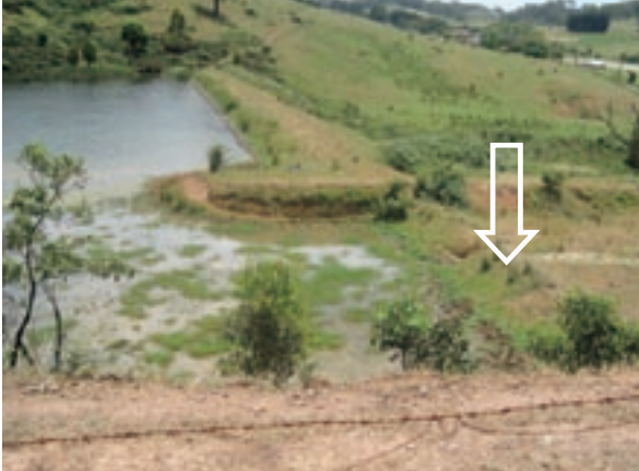
FIGURE 4. Dam No. 4 in 2007 showing the spillway still blocked by a mound of dirt, but now shrubs and vegetation are growing in the spillway and along the upstream face of the embankment.
