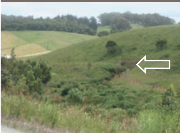
FIGURE 6. Dam No. 6 in 2007 showing the spillway still undercutting the dam wall. Dense vegetation is also now allowed to grow out of the embankment and to completely block the spillway.
