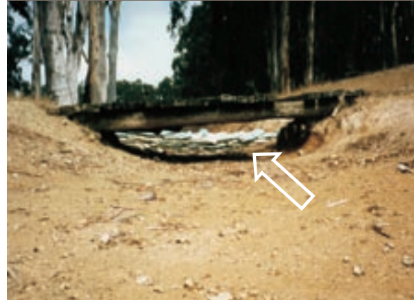
FIGURE 1. Dam No.2 in 1995 showing the spillway blocked by a walk-way bridge and sand bags, and trees allowed to grow out of the crest.
