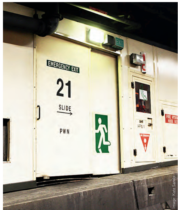
Impediments to evacuation. The jersey barriers had two small cut away steps (visible in bottom right of this photo) which the elderly participants were unable to use without assistance. They took around five seconds to climb the barriers with assistance.
